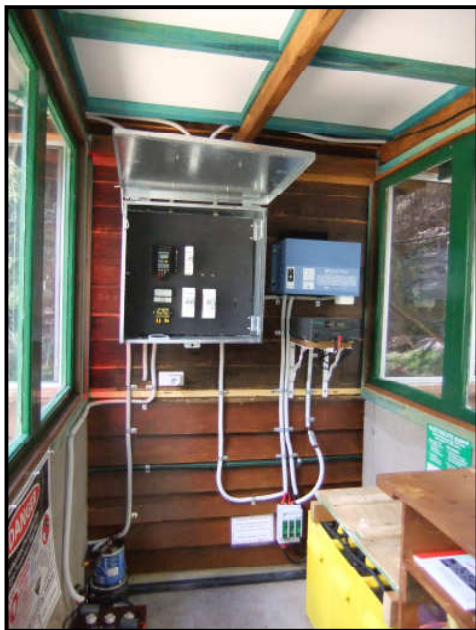
The inside of our new power/battery room.
